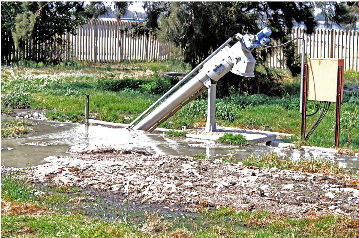
Above: The wastewater pump station in Seeiso Street, Sharpeville, is flooded with sewage, vandalised and abandoned.
