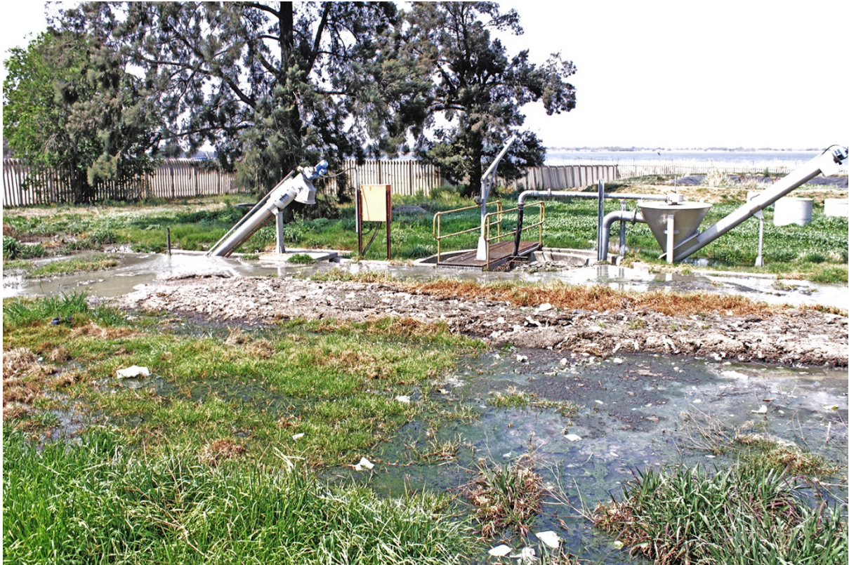
Above: The wastewater pump station in Seeiso Street, Sharpeville, is flooded with sewage, vandalised and abandoned.
