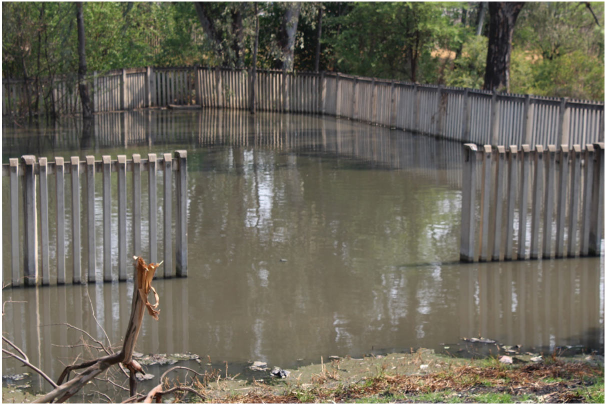
Above: The wastewater pump station in Golf Street, Three Rivers, Vereeniging is flooded with sewage and abandoned.
