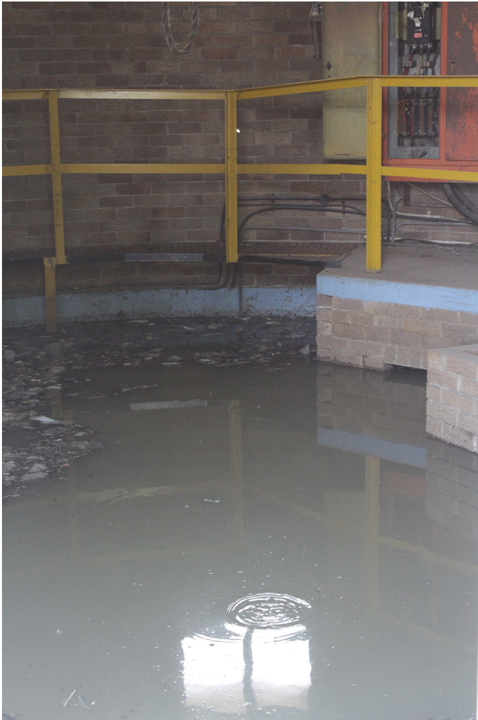
Above: The wastewater pump station in Seeiso Street, Sharpeville, is flooded with sewage, vandalised and abandoned.
