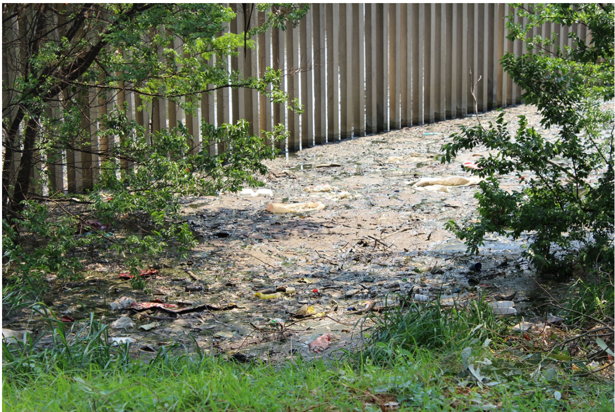
Above: The wastewater pump station in Golf Street, Three Rivers, Vereeniging is flooded with sewage and abandoned.
